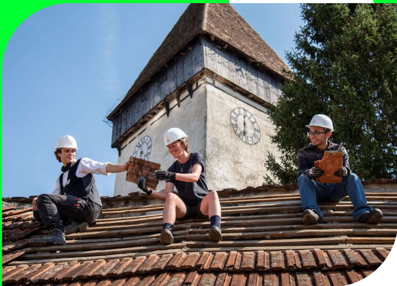
"Conservation works at the entrance area of a fortified church ensemble", Movile / Sibiu County, Romania © Maria Teresa Tenaglia / European Heritage Volunteers
