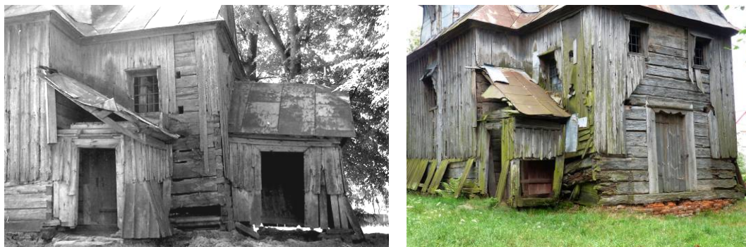
Fig. 5. Mięgisz Stary, progressive degradation of the church's construction structure: state in 1989 (left) and existing state in 2015. Source: photo by author
